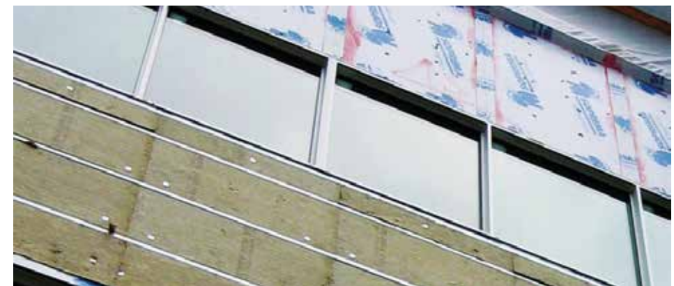
Exterior insulation installed in-between steel z girt cladding support attachment resulting in exterior insulation that is not continuous and does not meet energy codes (Source: Roxul, Inc.)
